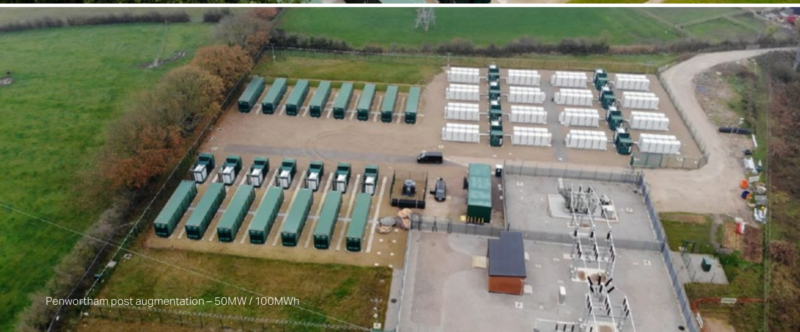
Penwortham pre augmentation – 50MW / 50MWh
